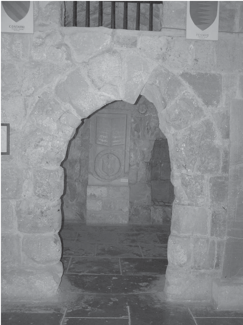
Fig. 26: Limassol Castle, lower level of cells, fire-damaged cell doorway [M. Olympios].
